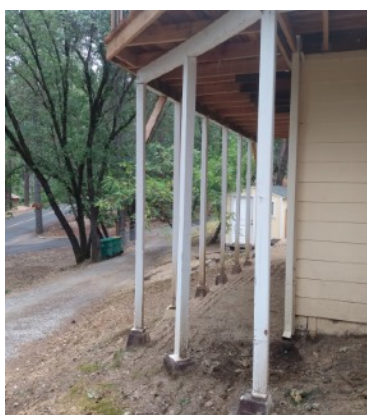
A great example of a deck with the space underneath kept completely clear, at a home having a recent assessment in our area.
